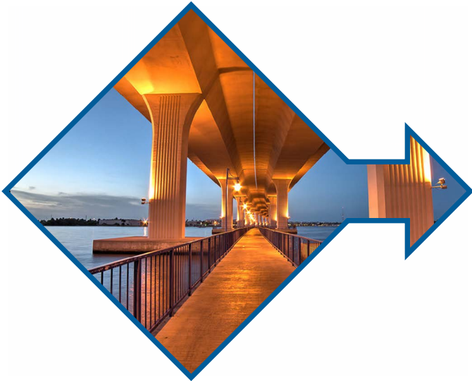
STRUCTURAL HEALTH MONITORING
